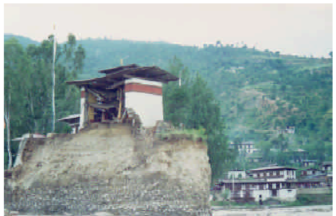
Plate 9.9: Damage caused by the flood of 1994 to one of the oldest and most sacred temples in Punankha. (Helvetas)
